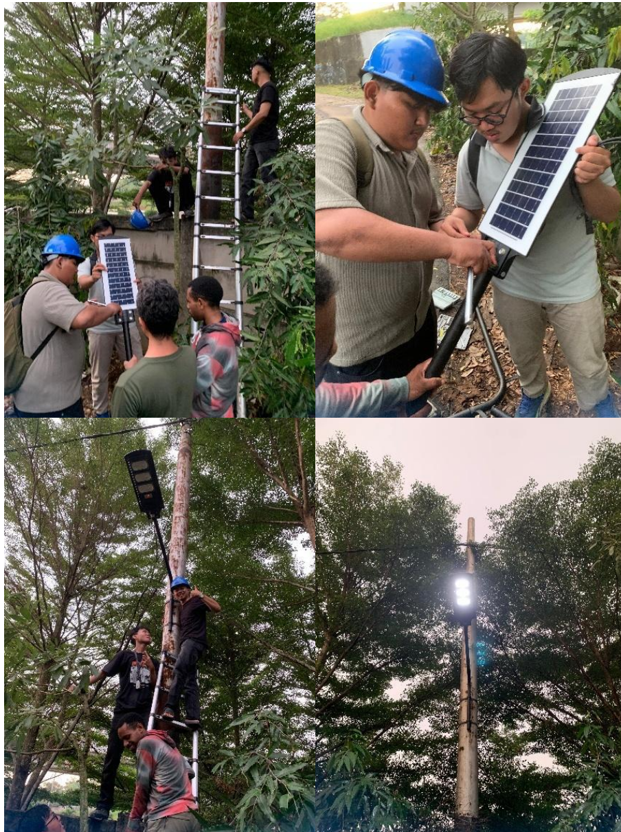
Gambar 2 Instalasi lampu panel surya
