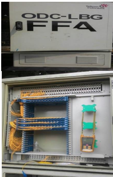
Gambar 2.1 Optical Distribution Cabinet
