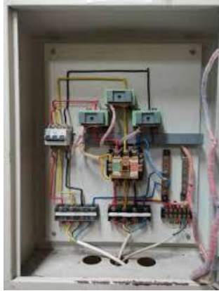
Gambar 1. Panel ATS ( Automatic Transfer Switch )
