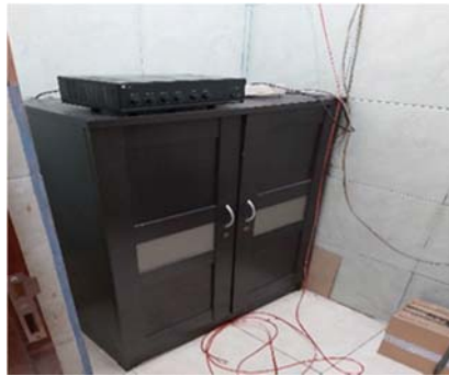
Gambar 1 Ruang Audio system
