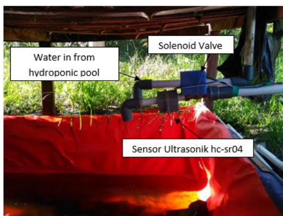
Figure 8. Ultrasonic sensor and solenoid valve at pond inlet.
